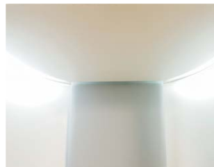
Controllable dimmed ceiling down lighting
